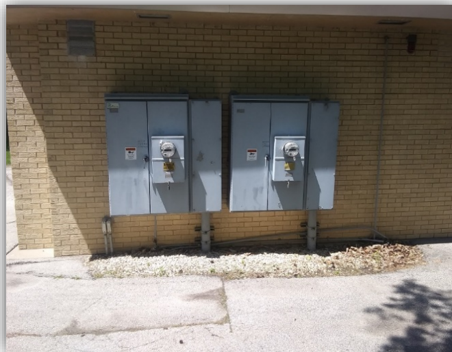
Building Metering Cabinets
