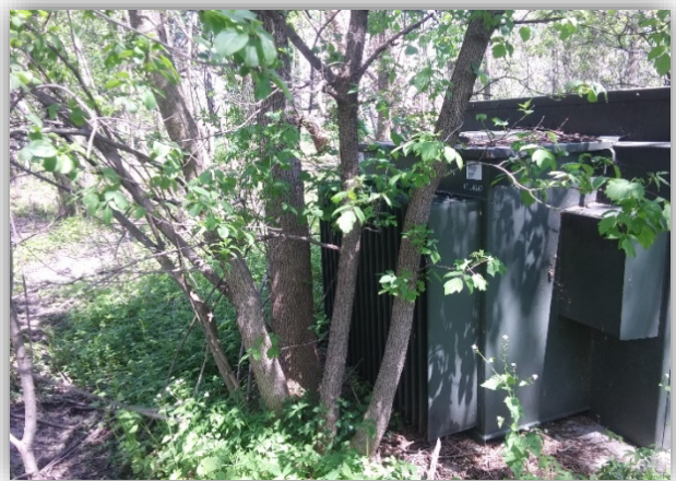
Normal Service Transformer (Facing North)
