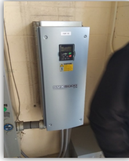
Pump 2 (125HP VFD)
