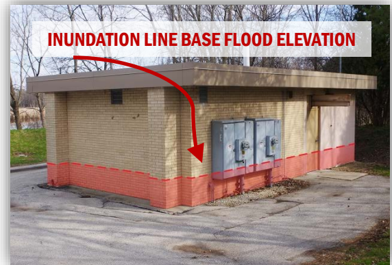
Lift Station E
