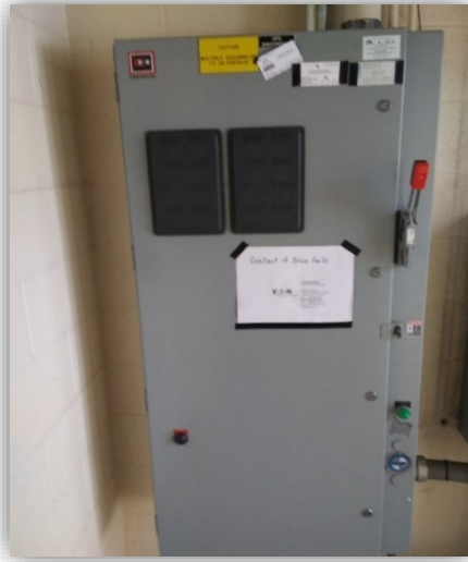
Pump 1 (50HP VFD)
