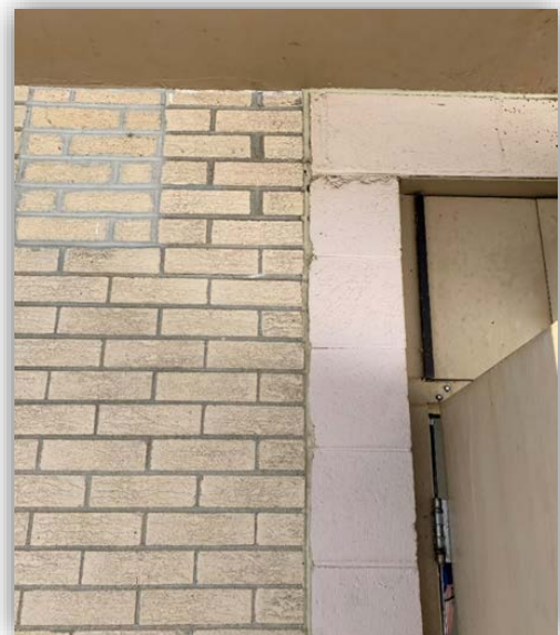
East expansion joint
