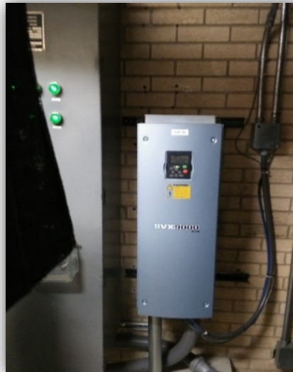
Pump 4 (125HP VFD)
