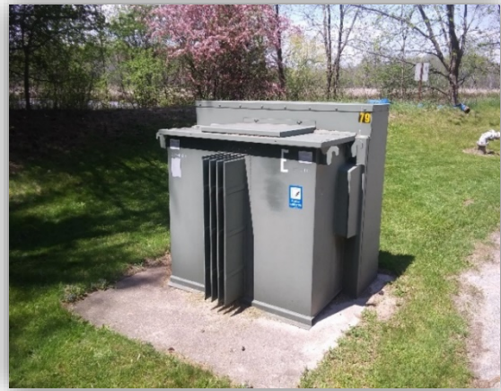
Standby Service Transformer (Facing South)
