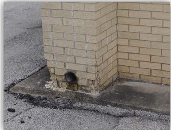
Brick damage at southwest bump out
