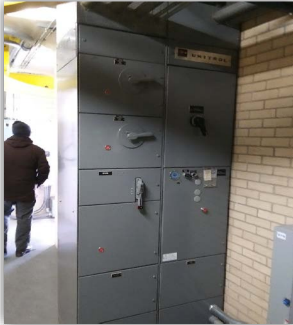
Motor Control Center
