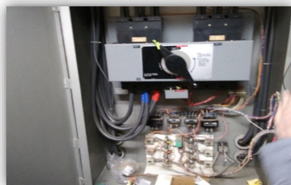
Automatic Transfer Switch (Door Open)
