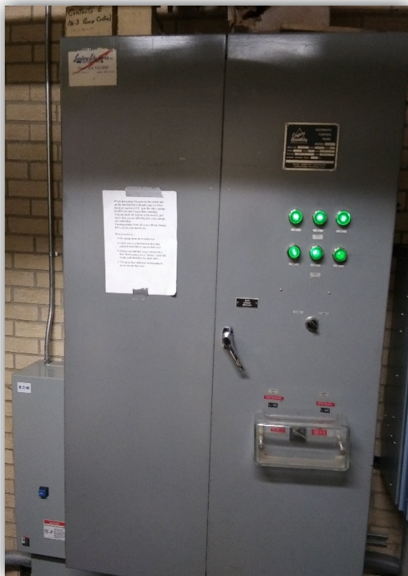
Automatic Transfer Switch (Front of Panel)
