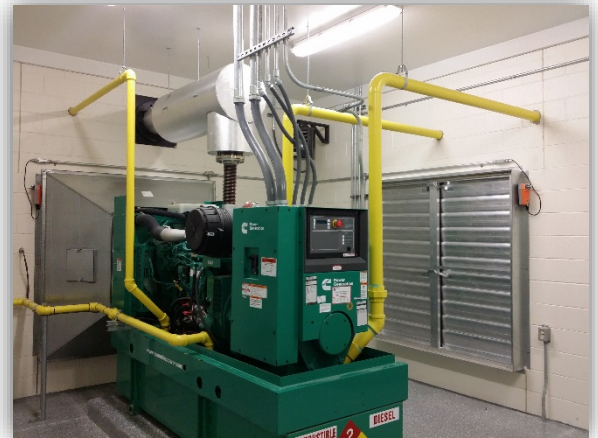
Example - 230 kW Generator
