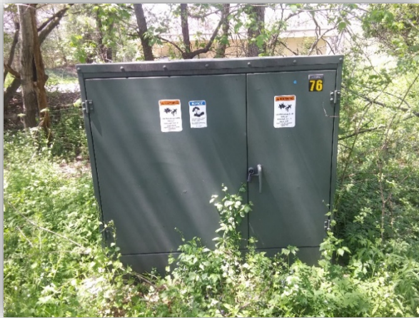
Normal Service Transformer (Facing South)
