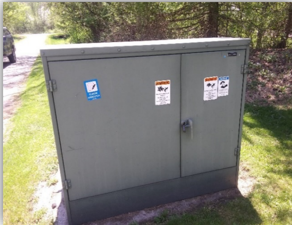
Standby Service Transformer (Facing North)
