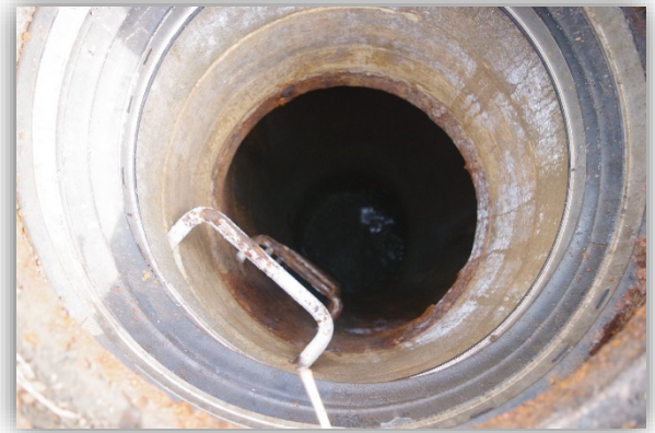
Influent sewer just west of lift station
