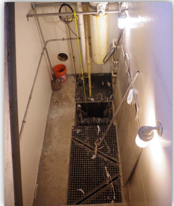
Station Wet Well
