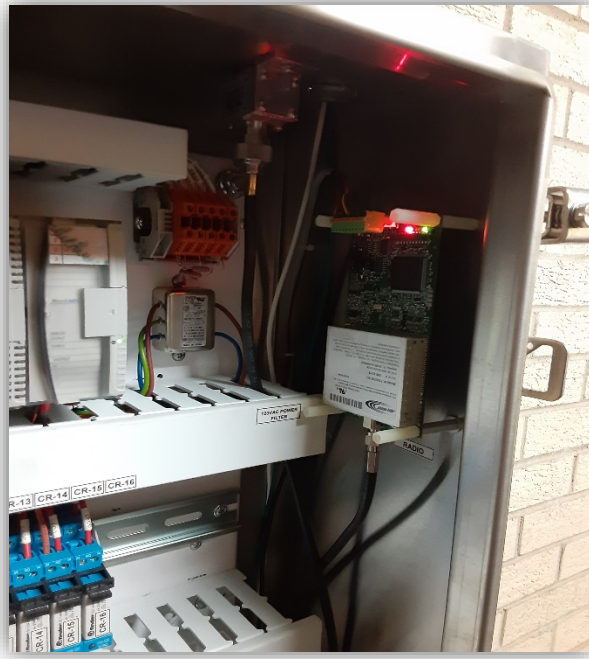
Pump Control Panel Radio (Door Open)
