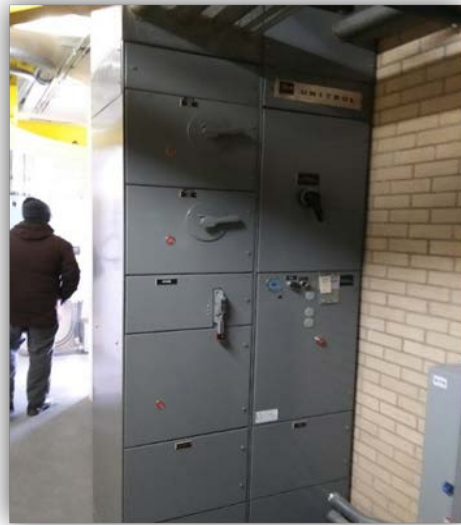
Pump 3 Constant Speed (125HP in MCC)
